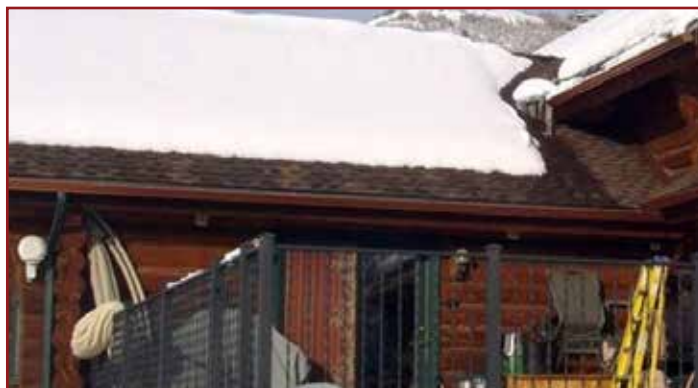
Heated roof valley and edges.
